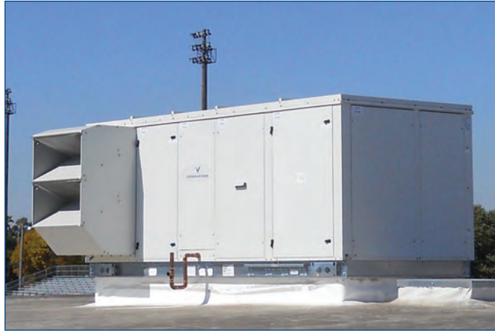
Energy recovery ventilators
