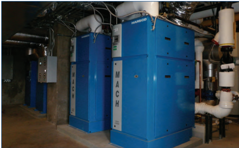
Boiler system upgrades meet Events Center demands
