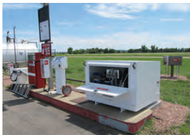
Vermillion Airport Fuel Dispensing Island with both old and new style dispensers, Vermillion, SD
