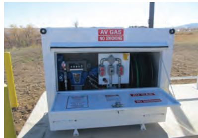
Avgas Dispenser at Sheridan County Airport, Sheridan, WY
